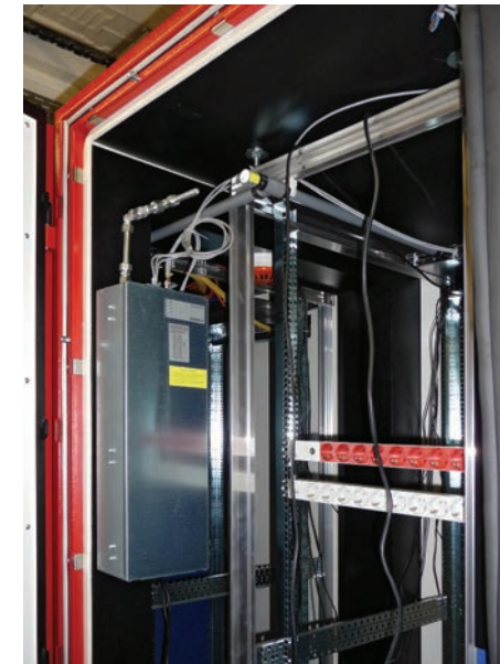
Internal Server Safe
